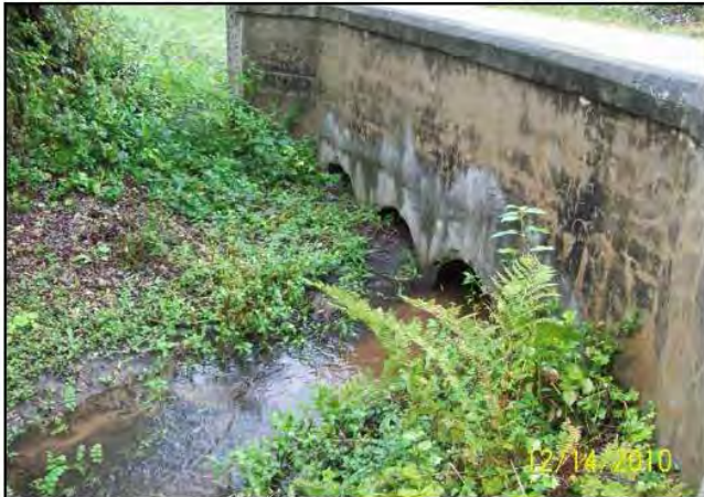
Photo 3. George Street bridge. Sediment and vegetation removal needed in the future. Bridge could also benefit from paint removal. (December 2010)
