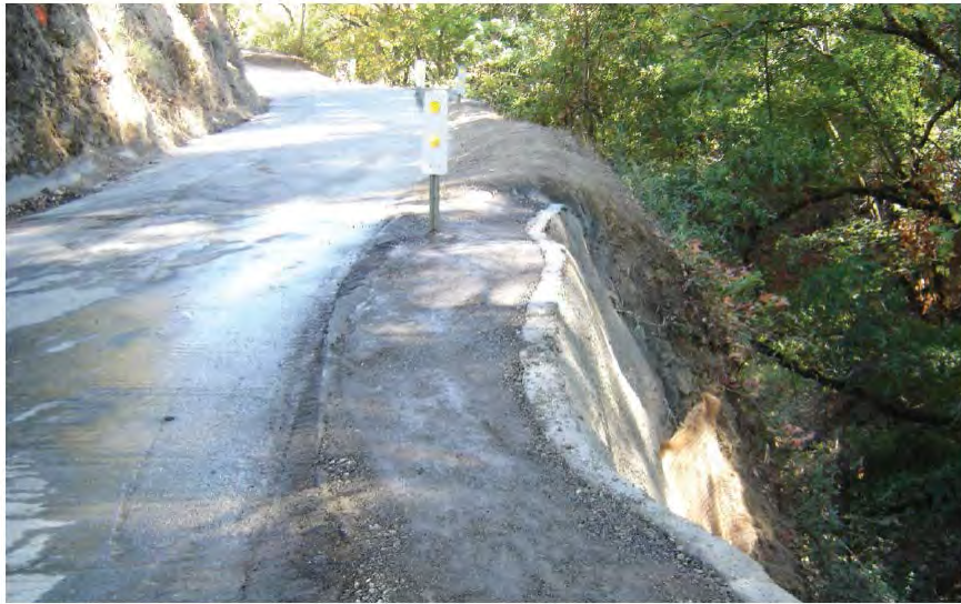
Photo 6. Example of a retaining wall at a bank stabilization site along Alpine Road. (October 2014)
