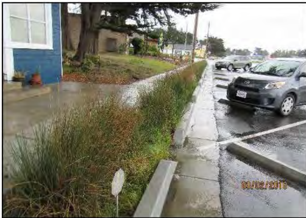
Photo 11. Bioretention swale along Carlos Street in Moss Beach that requires periodic vegetation removal, light sediment clearing, and planting. (March 2018)
