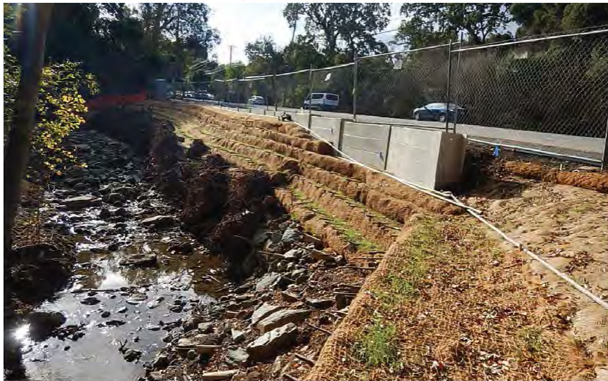
Photo 7. Example of a soldier pile wall fronted with rock, rootwads, and vegetation following installation at Los Trancos Rd. (November 2017)
