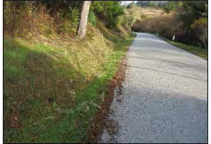
Photo 14. Another example of an inboard unpaved ditch along Gazos Creek Road. (December 2019)
