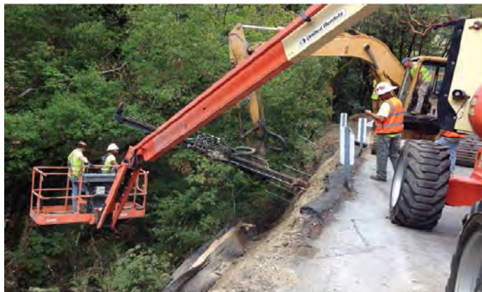
Photo 5. Example of soil nailing at a bank stabilization site along Alpine Road. (September 2014)
