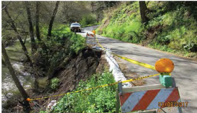
Photo 3. Example slope failure along Gazos Creek and Gazos Creek Road. This site was addressed in the County's 2017 emergency permit application. (March 2017)
