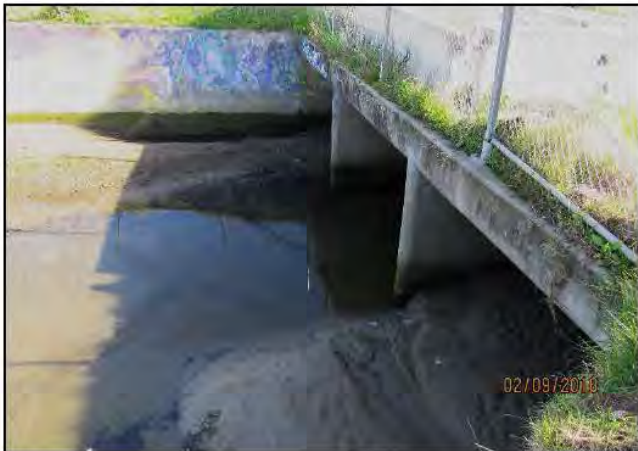
Photo 5. Sediment removal needed at the San Bruno Creek and Walnut Street crossing. (February 2018)
