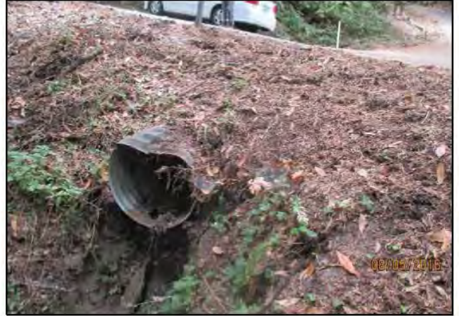
Photo 2. Deteriorated CMP culvert on Alpine Creek that requires replacement. (August 2016)
