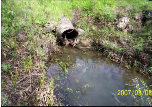
Photo 1. Deteriorated corrugated metal pipe (CMP) culvert located at Pigeon Point Road that requires replacement. (March 2007)
