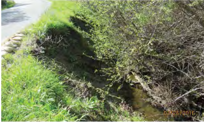
Photo 2. Bank failure along Lower Bear Gulch Road and adjacent to Clear Creek, an Intermittent tributary to San Gregorio Creek. (February 2016)
