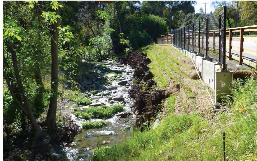
Photo 8. Example of a soldier pile wall with grown-in vegetation at Los Trancos Rd. (March 2018)
