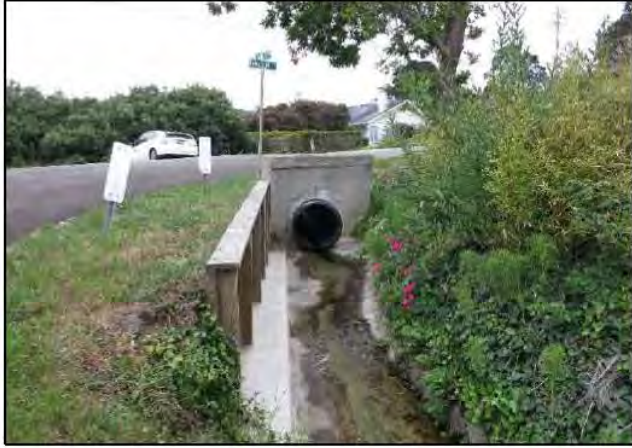
Photo 7. Paved ditch downstream of Farallone Avenue and Kanoff Street in Montara. Ditch is routinely maintained with a Vac-Con truck. (May 2015)
