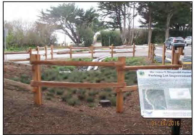
Photo 12. Bioretention swale at the Fitzgerald Marine Reserve parking lot, which requires periodic vegetation removal, light sediment clearing and revegetation. (January 2016)
