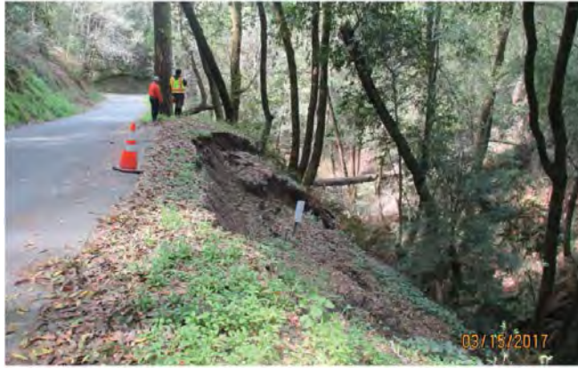
Photo 1. Example slope failure above unnamed tributary to Alpine Creek. This site was addressed in the County's 2017 emergency permit application. (March 2017)
