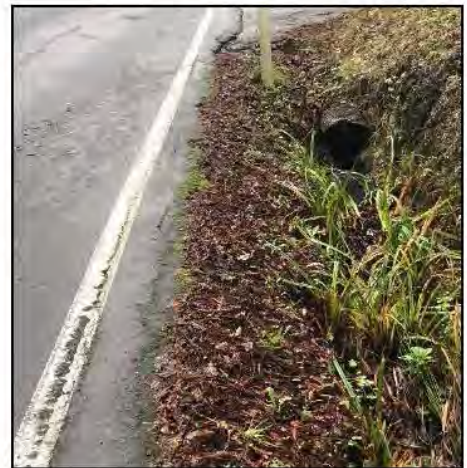
Photo 16. Example of an unpaved ditch and roadside culvert along Pescadero Creek Road and entrance to Sam McDonald Park. (December 2019)
